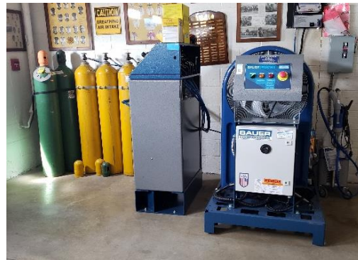
Air Compressor and Cascade System
