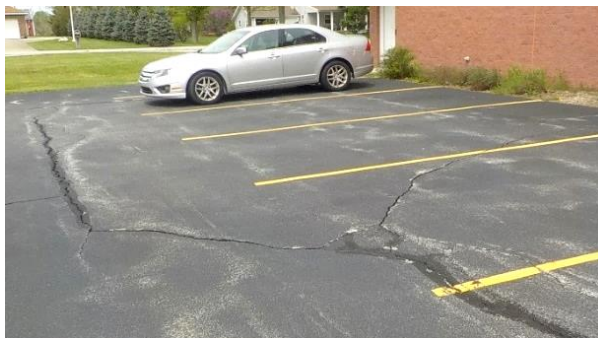
Cracks in Asphalt - West Parking Lot
